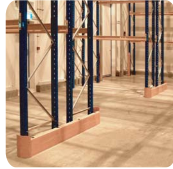
Double deep racking to maximise space
